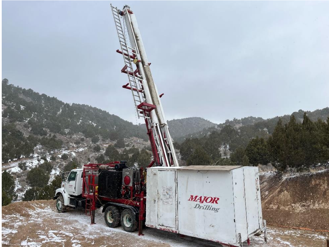
Figure 1: Diamond drill rig to test potential copper-gold porphyry mineralization set up at the Big Hill target at Tintic Project (December 2023)
