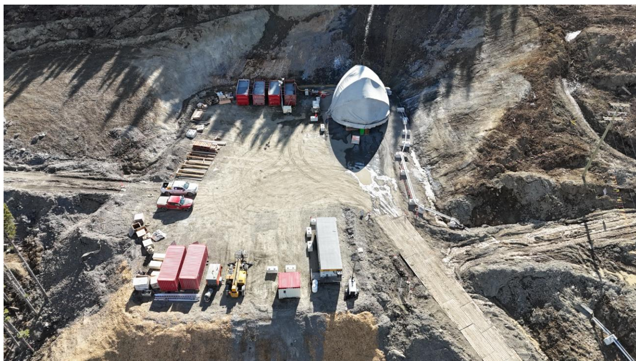
Figure 5: Lowhee Zone ventilation raise bore.
