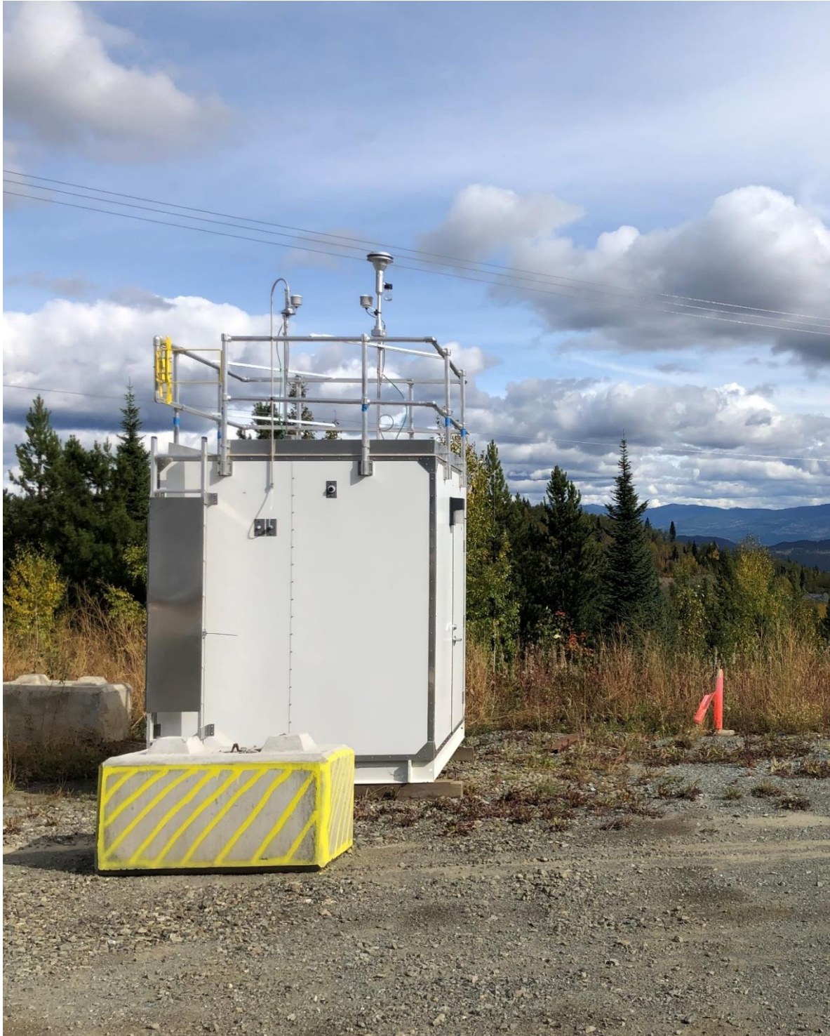
Figure 3–3: Photo of QR Mill Air Quality Monitoring Station
